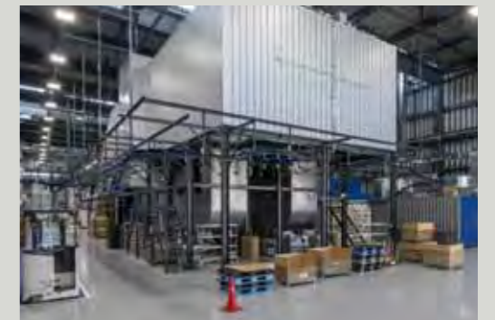
Powder coating equipment (Hakusan Factory)
